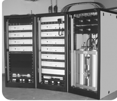
Figure 7-2 MX800's Setup in system rack
